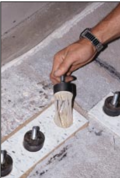
Figure 4. Even though the adhesives had cured for three days, pull-off tests revealed many were still gummy or tacky, forming the adhesive strings shown.
